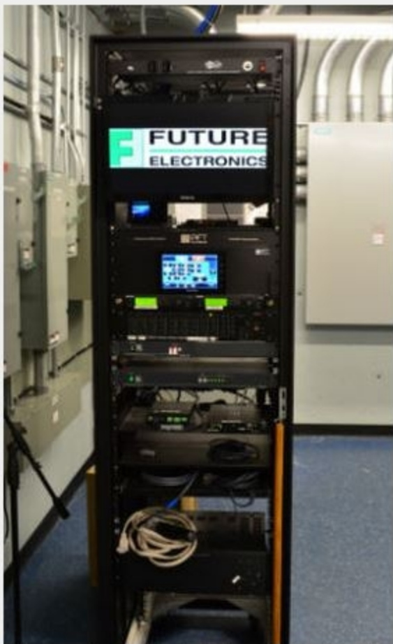
The main rack at Future Electronics consists primarily of a control system, IP video gateway, video matrix, audio AEC DSPs, audio recorder, microphone receivers with an antenna distribution system, preview monitor and television receivers.
